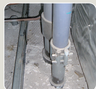
▲ PVC + Steel Pipe Connection
