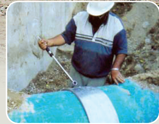
▲ UK: buried water supply pipes
