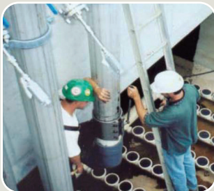
▲ Canada: water purification facility
